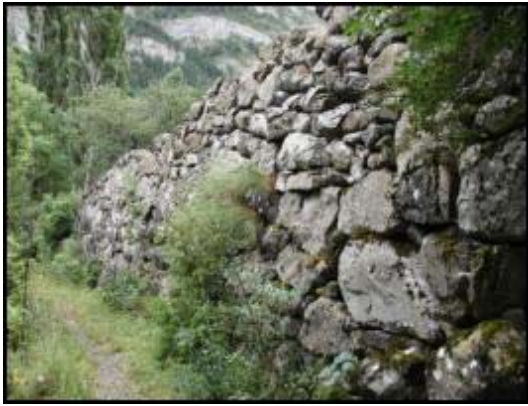
Figure 2.3. Actual state of "Neighbours wall"
